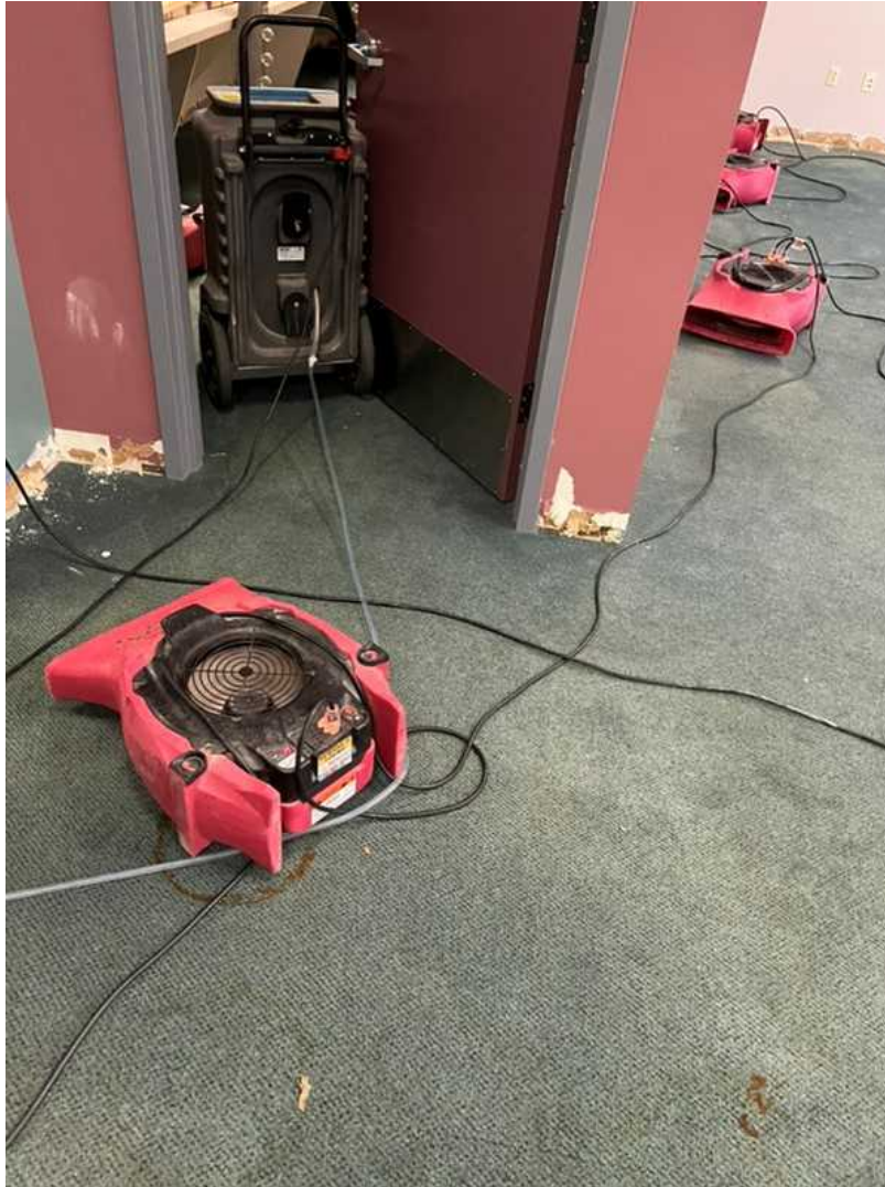
20 25-12-30-22 (92) Date Taken: 12/31/2022 Equipment in room 1 and Storage area
